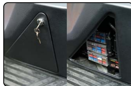
New fuse panel providing service accessibility
